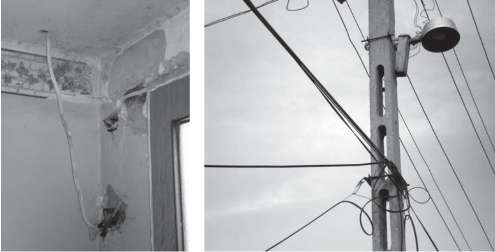
Figure 16. Individual Solutions to Access Electricity in Tatabánya's Mésztelep
